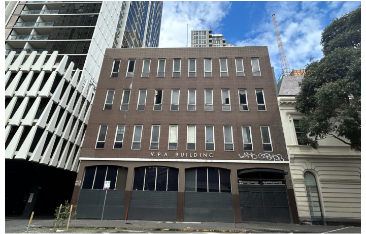
Figure 18: Close-up of the Victoria Police Association Building, with smashed windows. Erica Cervini, 2025.
